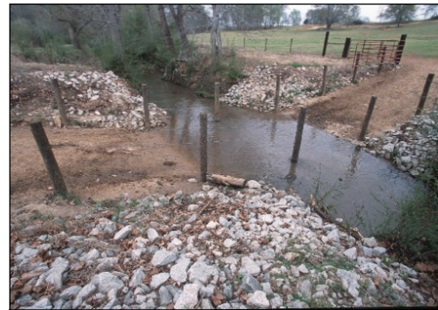
Concrete water crossing for livestock. Photo by Jeff Vanuga, NRCS.
