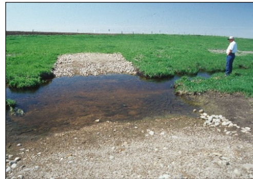
This livestock crossing was installed to offer a stable point for livestock to cross a stream. This low cost engineering practice is an efficient method of reducing bank erosion. Photo by Don Poggensee, NRCS.
